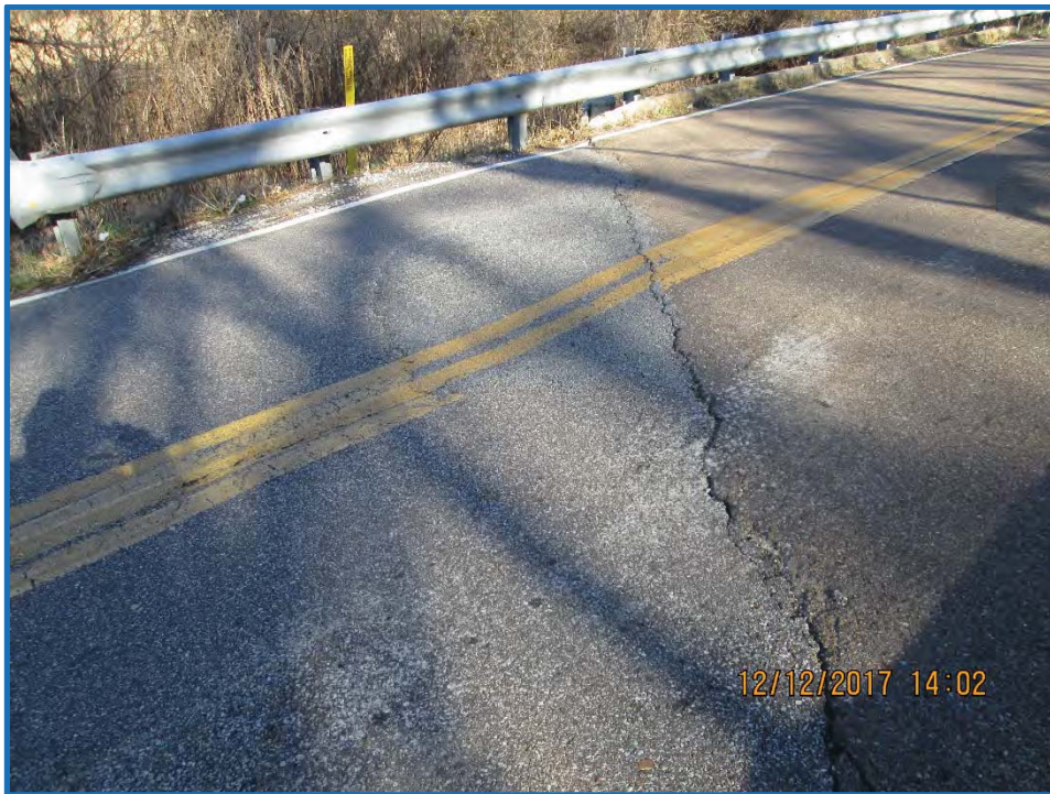
Pavement failure at west end of bridge
